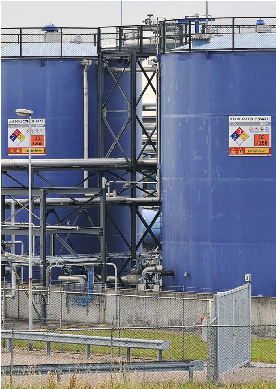
PGS 29 tanks in Gaag (foto SodM)
