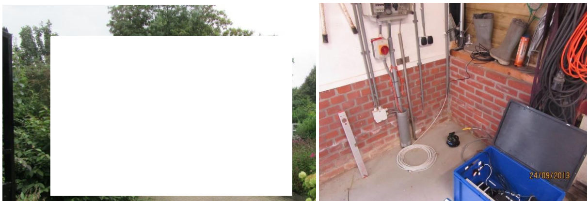
Figure 2.14a: Shed with BWIR and 2.14b: photo of the accelerometer inside the shed
