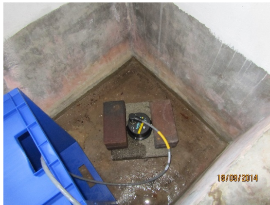
Figure 21. An inappropriate sensor mounting from BWIN station
