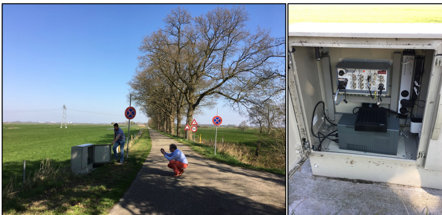
Station G710 Photos. Left: Overview of site. Right: Inside G710 box, showing 3 channel Obsidian datalogger, strong motion sensor located underneath the datalogger as at G39.
