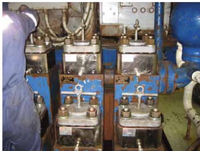
Mud pomp (foto SodM)
