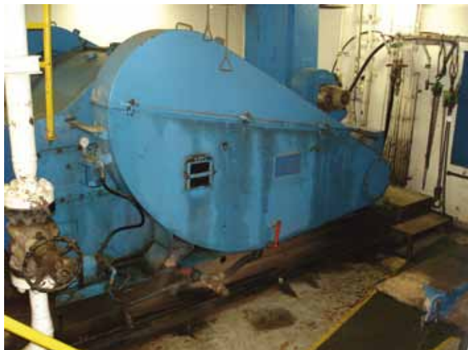
Mud pomp (foto SodM)
