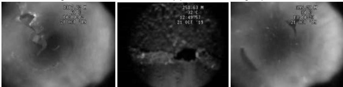
Figure 3. Observations from downhole camera run in 2 ⅞" tubing. Collapsed tubing at HUD (left), Hole in tubing at ca. 250m (middle), 2 holes across each other at ca. 395m (right)
