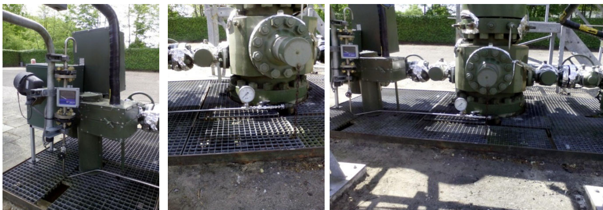
Figure 2: Venting Assembly installed at ROW-7.
