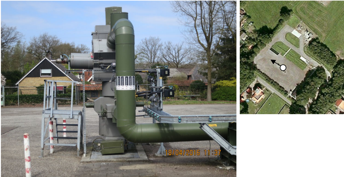
Figure A2.3: Well head of well ROW2 (right) at ROW2 site. Taken north of well looking to west site boundary (indicated by point and arrow on aerial photo).
